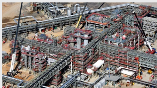
Photo: Chevron advanced construction on the alkylation retrofit project at the Salt Lake City Refinery during 2020.
