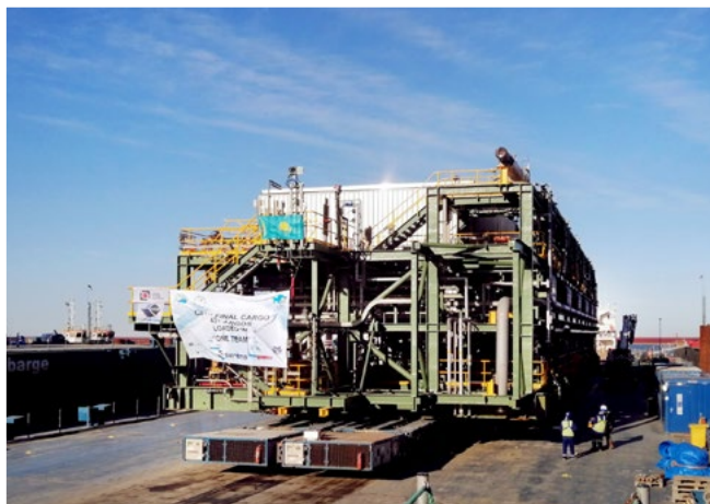
Photo: Progress continued for FGP/WPMP, including sealift transportation of the final module during 2020.
